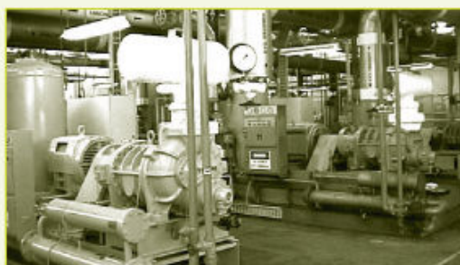
Plant room showing screw compressors
